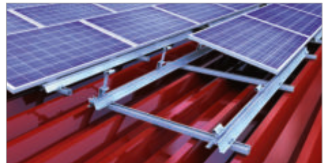
Clamping system: South-facing on east-west roof
