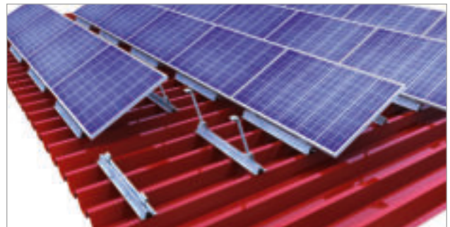
Clamping system: South-facing
